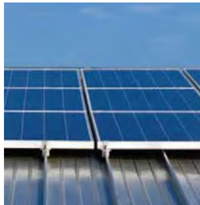
Roof mounted photovoltaic (PV) arrays
